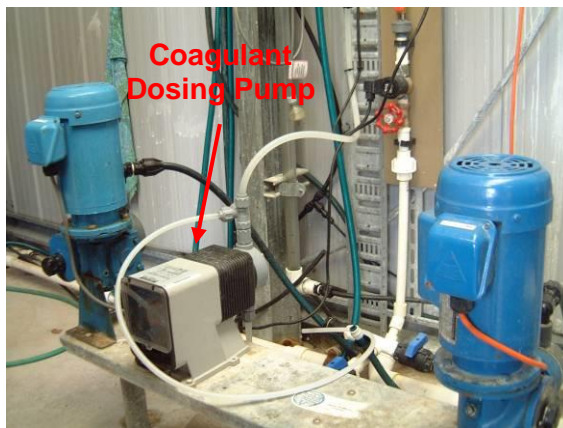
Photo of Coagulant Dosing Pump
