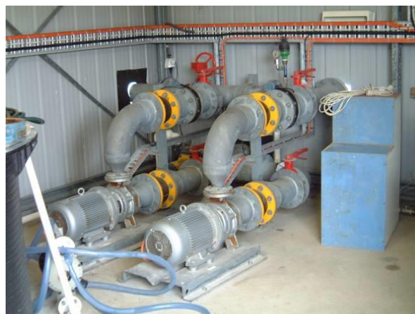
Photo of High Lift Pumps
