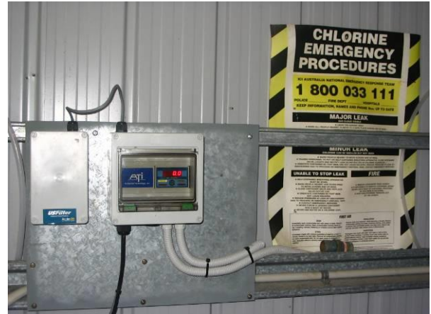
Photo of Chlorine Leak Alarm Panel
