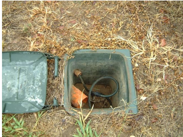
Photo of Coagulant Dosing Valve Pit at Dosing Point
