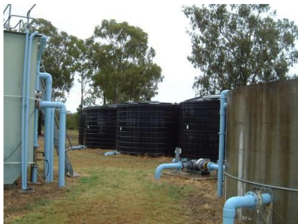
Photo of Clear Water Storage Vessels
