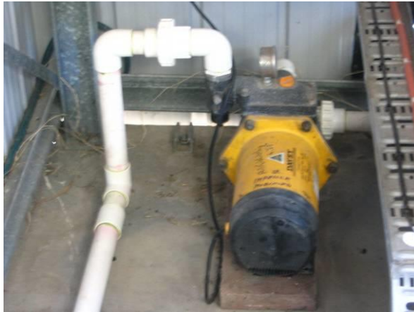
Photo of Chlorine Booster Pump
