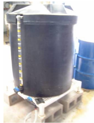
Photo of Coagulant Storage/ Dosing Tank and Drums
