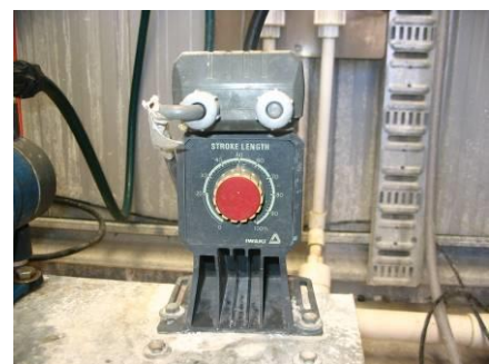
Photo of Lime Dosing Pump
