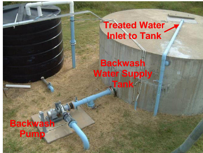
Photo of Backwash Water Supply System
