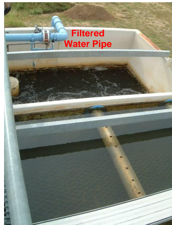
Photo of Filter and Clarifier (Top View)
