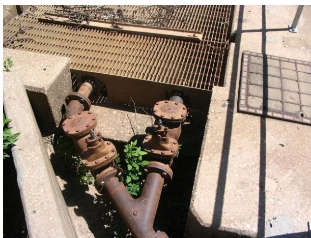
Photo of Raw Water Pump Pit and Pump Isolation Valves
