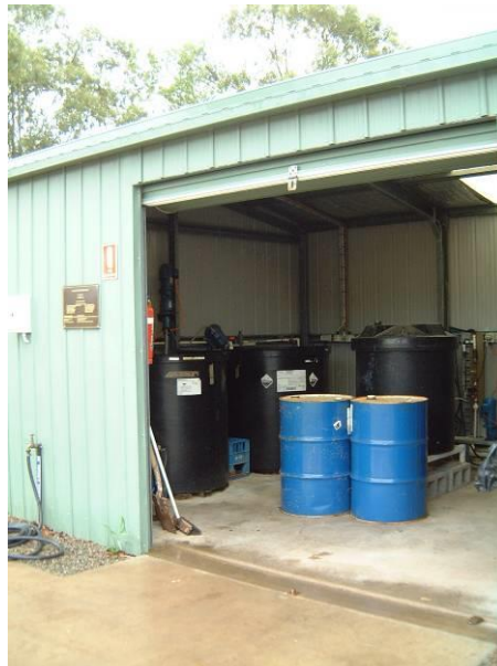
Photo of Chemical Tanks in Storage Shed
