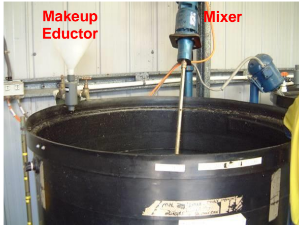
Photo of Polyacrylamide Mixing/Dosing Tank
