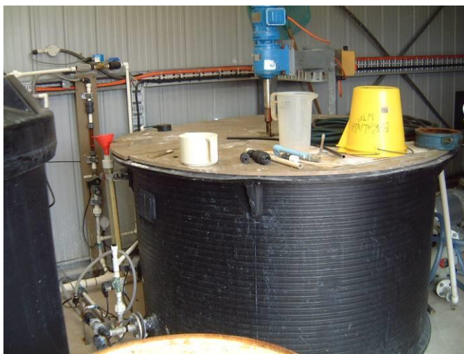
Photo of Lime Dosing Tank
