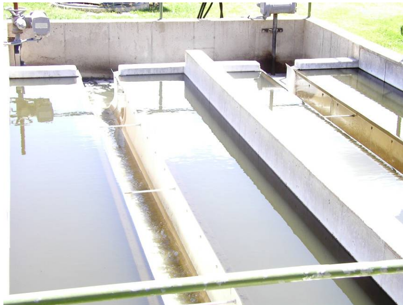
Figure 5.9: Sand filters in operation opposite to operational specifications.
