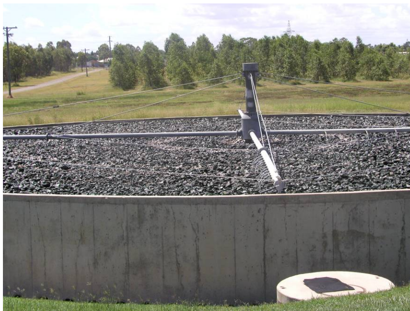
Figure 5.5: Trickling filter at Biloela that was on line at the time of the site visit.
