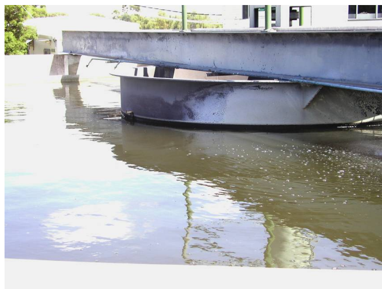
Figure 5.8: Secondary Clarifier at Biloela STP, some bubbles on surface, indicating some denitrification.
