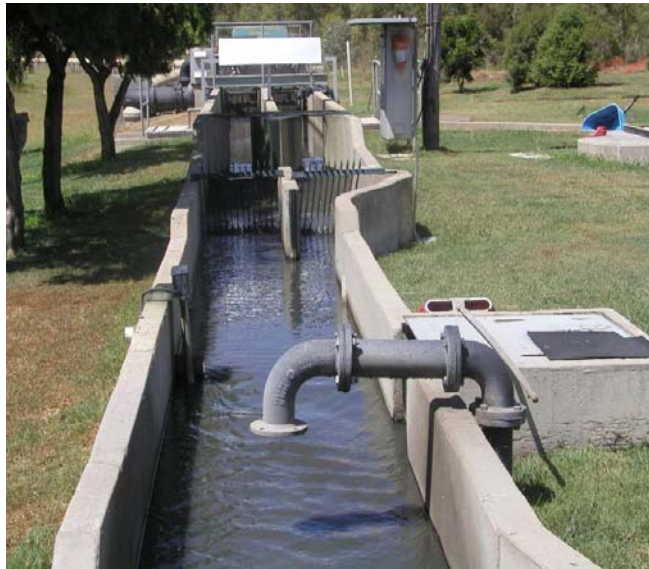
Figure 5.3: Grit channels for the Biloela STP
