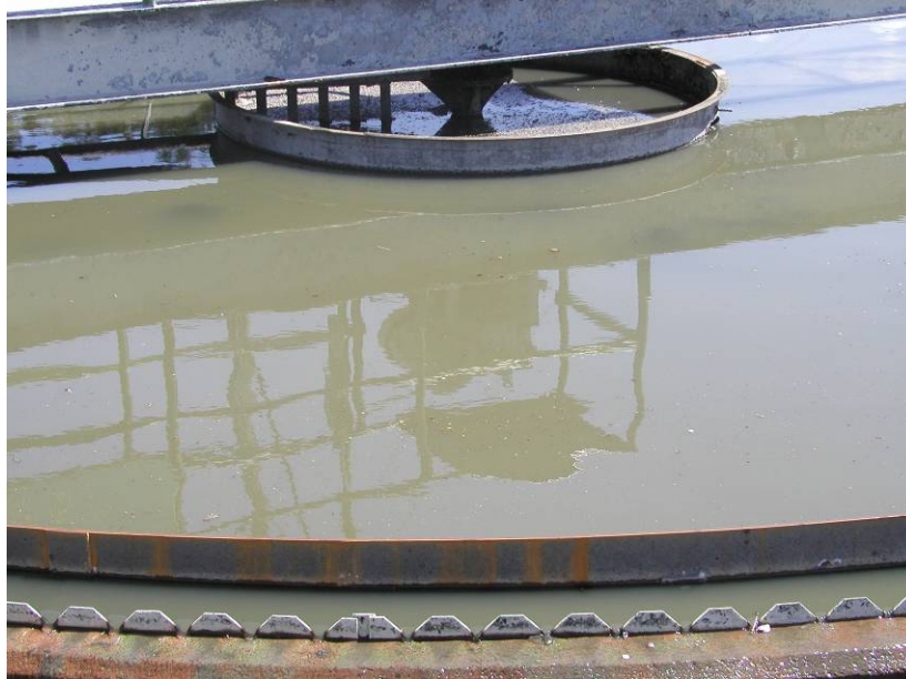
Figure 5.4: On line Primary Sedimentation Tank
