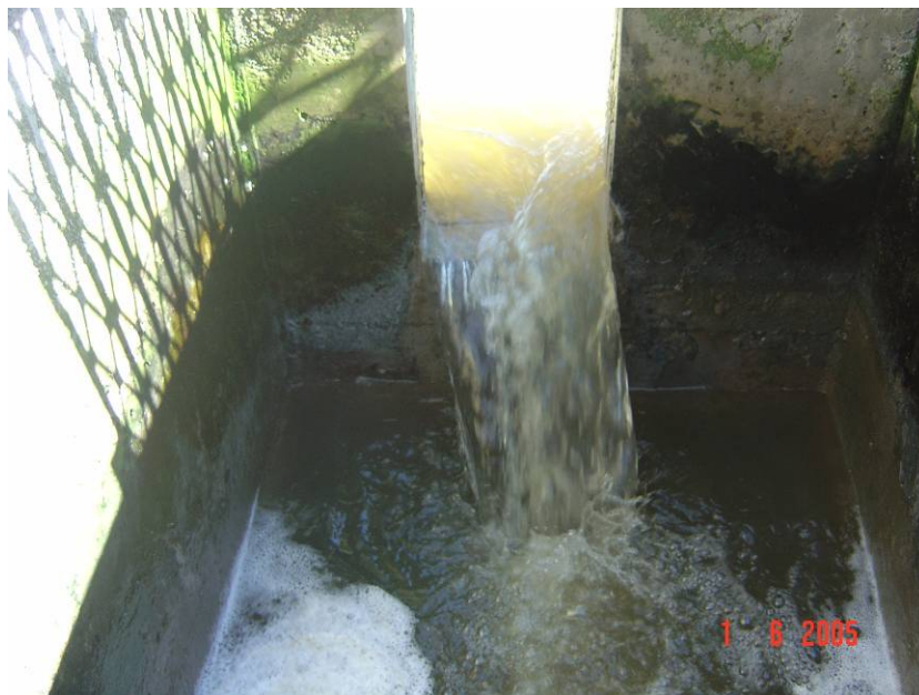
Figure 5.7: Uneven flow into the inlet feeding chamber for trickling filter one (current off line filter)
