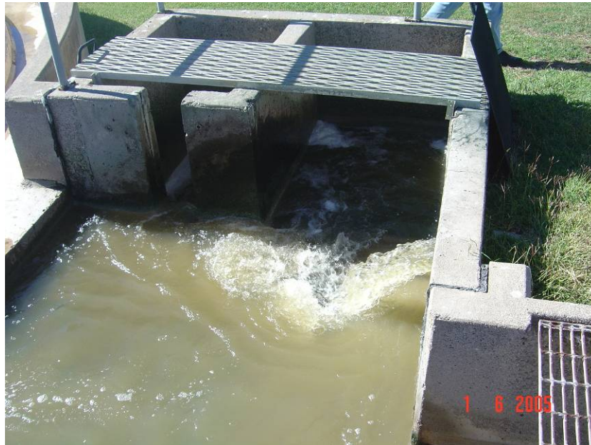
Figure 5.6: Inlet distribution well for the trickling filters showing the recirculation flow entry point.
