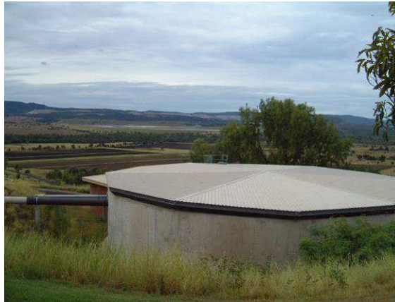
Photo of Clear Water Storage Tank
