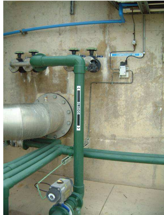
Photo of Automatic Sludge Bleed Valves
