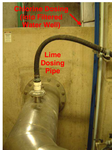
Photo of Post-Lime and Chlorine Dosing Points
