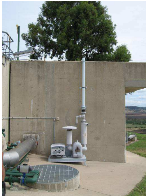
Photo of Aeration Blower at Flash Mixing Tank
