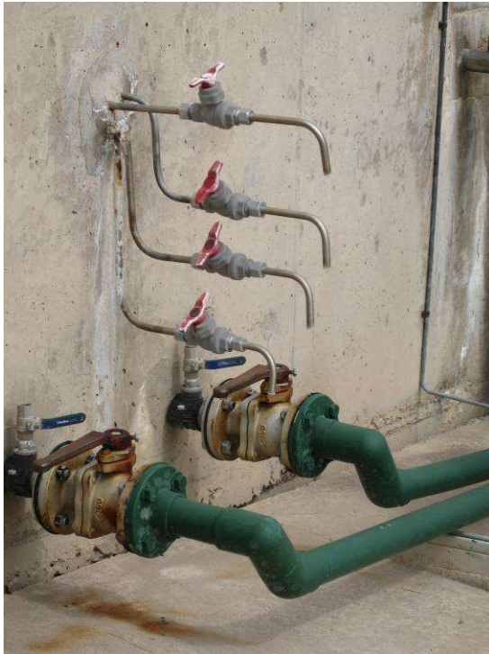
Photo of Sludge Testing Valves and Manual Sludge Bleed Valves
