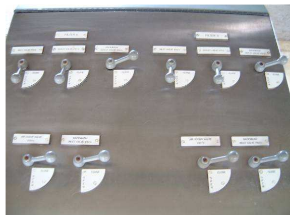
Photo of Filter Valves Control Panel
