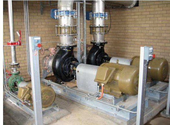
Photo of Backwash Pumps
