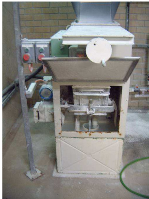
Photo of Lime Screw Feeder and Dilution Tank
