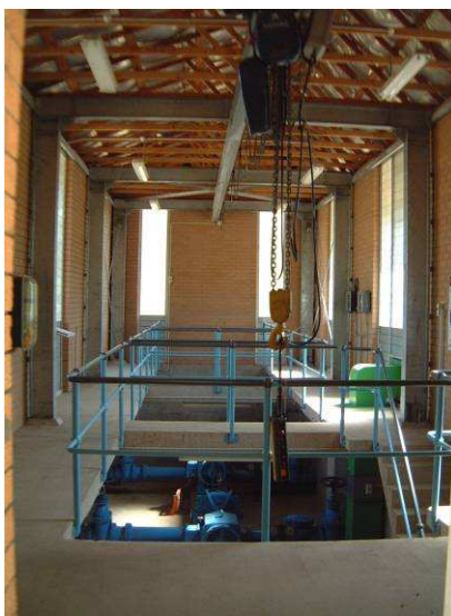
Photo of Raw Water Pump Station
