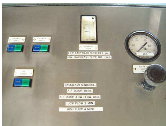
Photo of Main Backwash Control Panel
