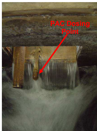
Photo of Normal PAC Dosing Point in Filter Inlet Channel
