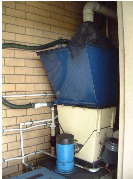
Photo of PAC Dosing System
