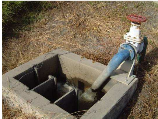
Photo of Lagoon Wastewater Splitter Box
