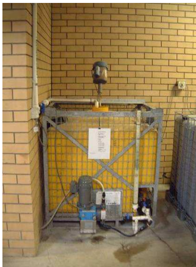
Photo of Cationic Polydadmac Dosing System
