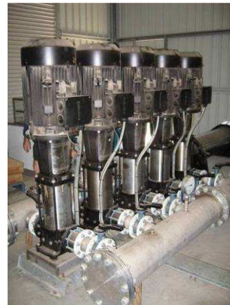
Photo of Treated water pressure pumps
