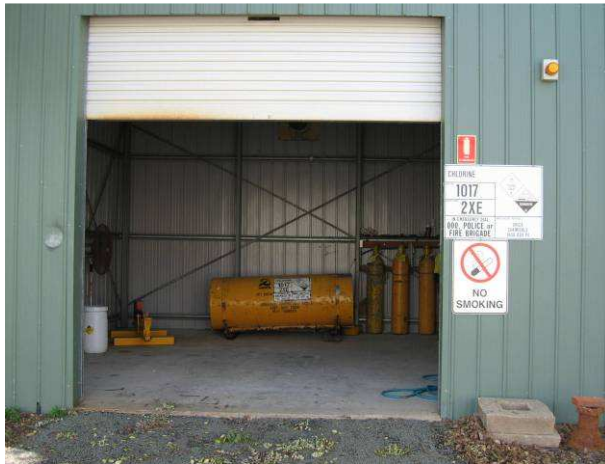
Photo of Chlorine Room
