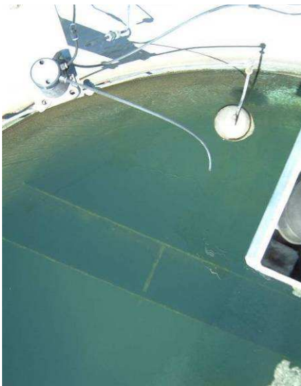
Photo of Stage 2 Filter Showing Level Switches
