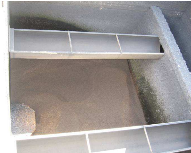
Photo of Stage 1 Filter Showing Uneven Media and Concrete Etching
