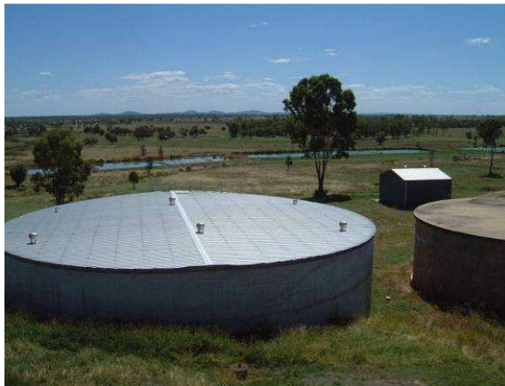
Photo of Clear Water Tanks
