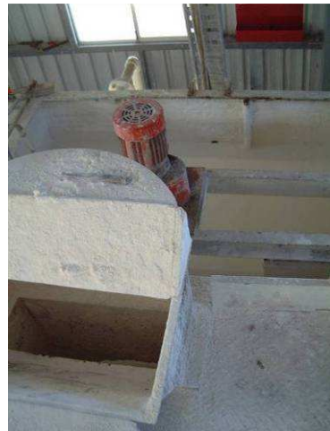
Photo of Lime Unloading Chute
