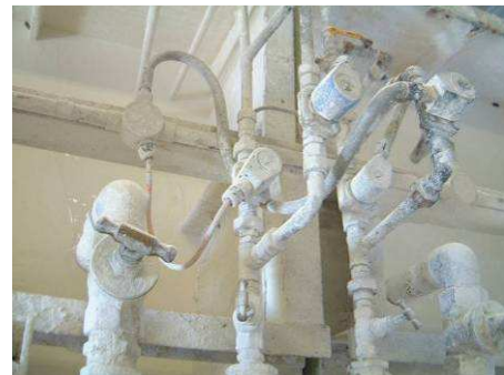
Photo Showing Dilution Water and Flush Lines for Lime System
