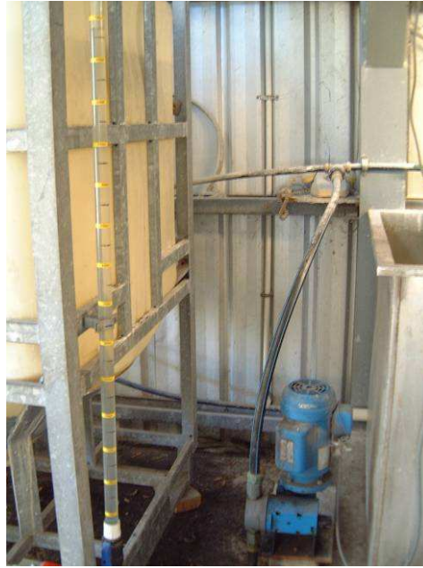
Photo of Nalco Dosing Pump
