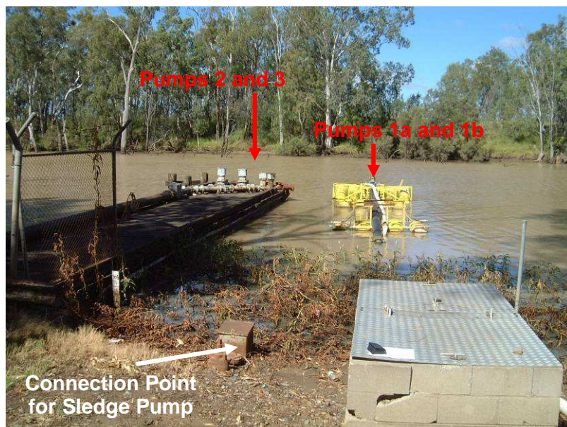
Photo of Pumping Facilities at River
