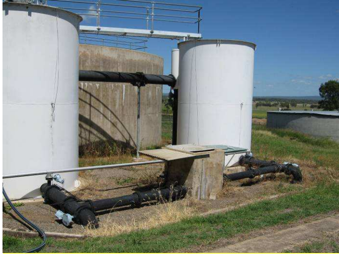
Photo of Filtered Water Weir Box Where Stage 1 and 2 Filtered Waters Blend
