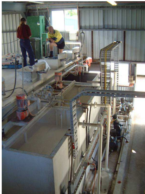
Photo Showing Unguarded Chemical Dosing Platform
