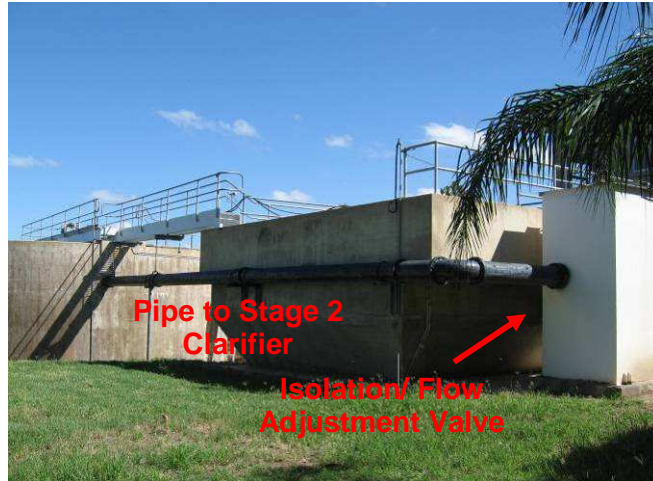
Photo Showing Connection From Flash Mixing Tank to Stage 2 Clarifier
