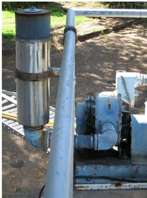
Photo of Blower for Aeration of Flash Mixer
