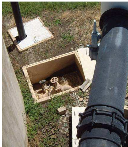
Photo of Stage 2 Clarifier Sludge Bleed Controls
