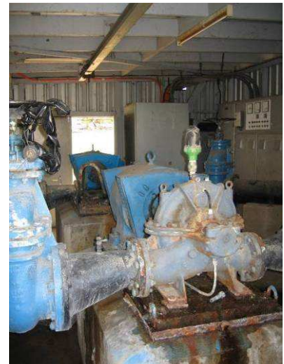
Photo of Backwash Pumps
