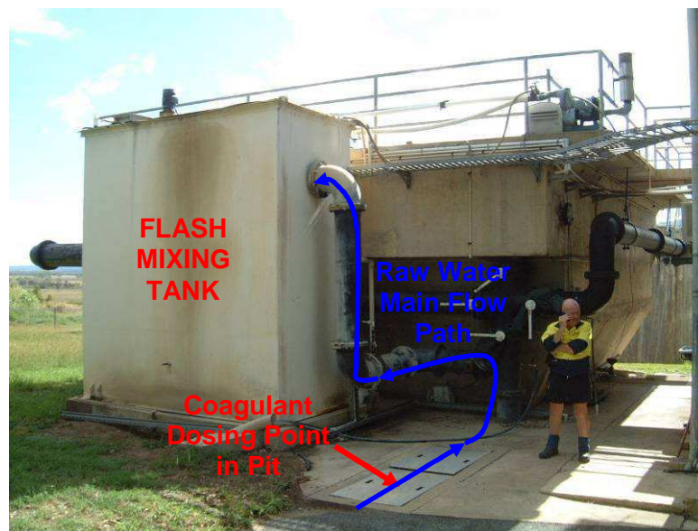
Photo of Nalco Coagulant Dosing Pit on Raw Water Main
