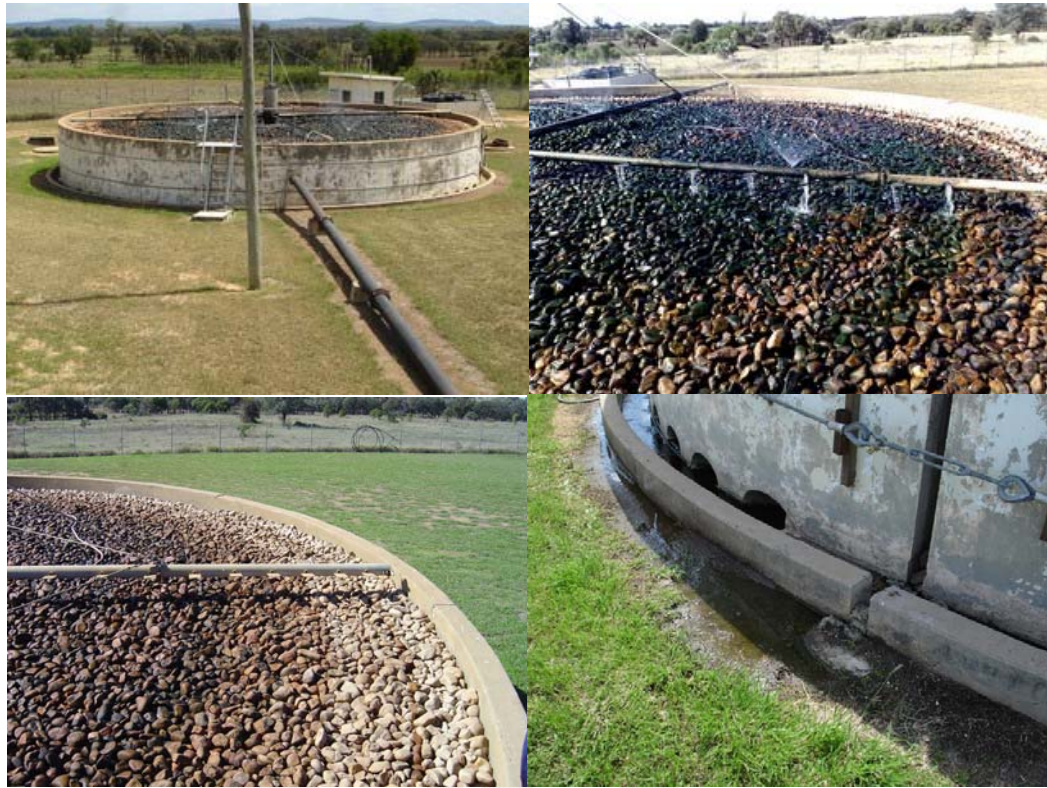
Figure 5-4: Trickling Filter at Taroom
