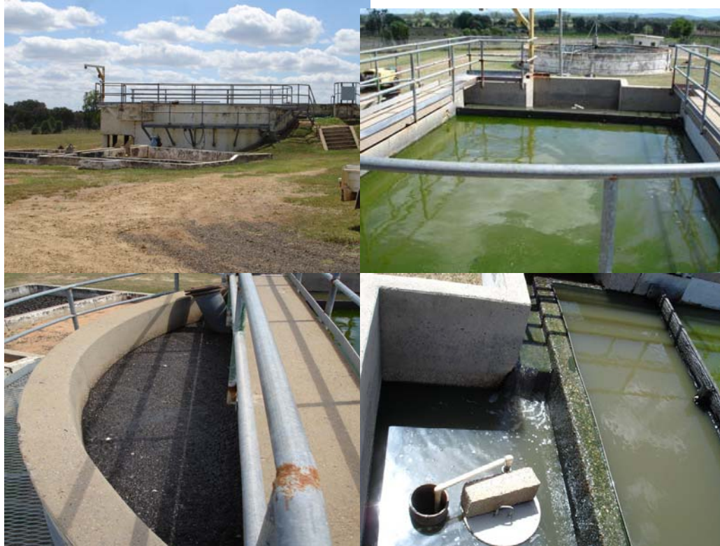
Figure 5-3: Imhoff Tank at Taroom
