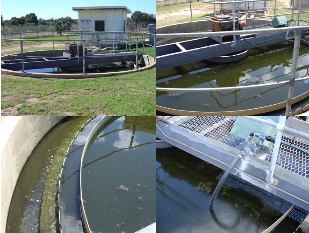
Figure 5-2: Humus tank at Taroom STP.
