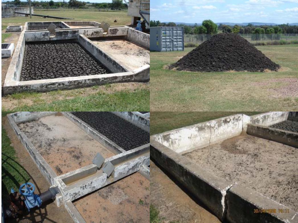
Figure 5-4: Sludge drying beds at Taroom
