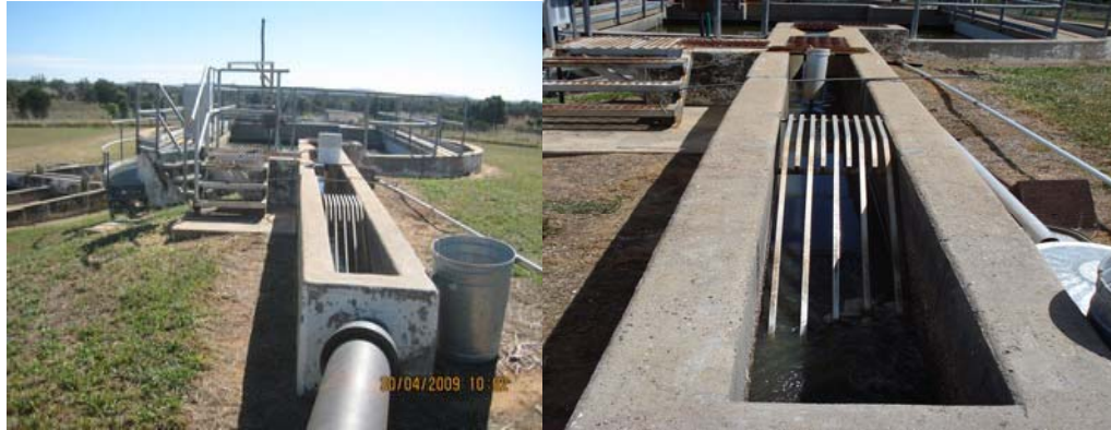
Figure 5-1: Inlet Works at Taroom
