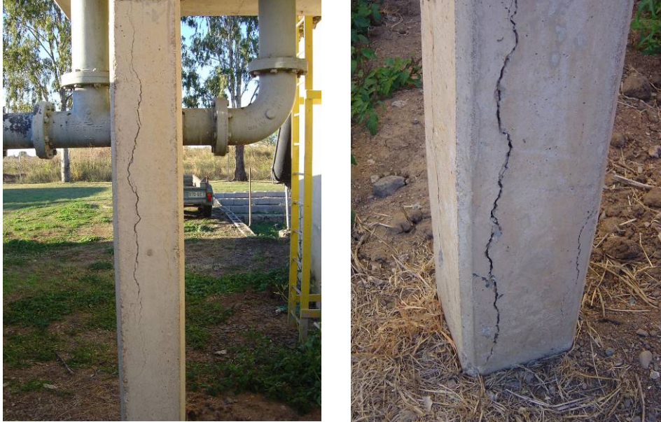
Figure 6-2: Cracks in supporting legs of Imhoff Tank
