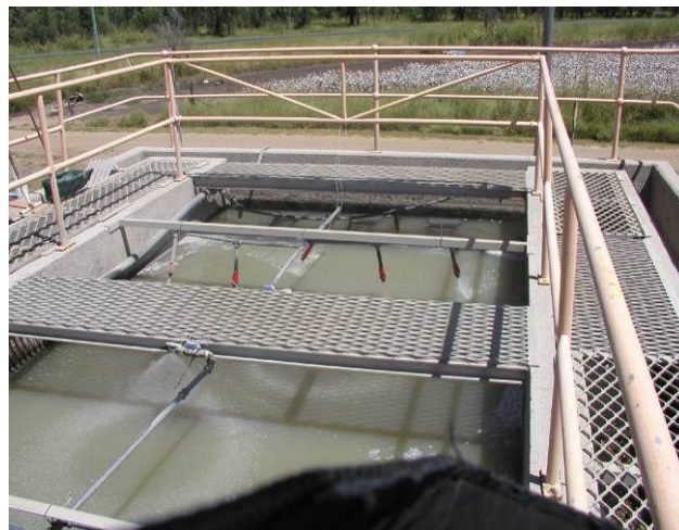
Figure 6-1: Surface of Imhoff tank at Theodore STP
