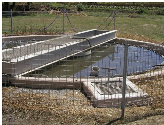
Figure 6-4: Humus tank at Theodore STP.
