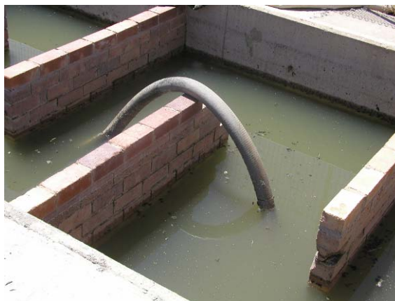
Figure 6-5: Chlorine Contact Tank
