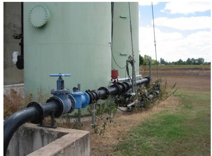
Photo of Backwash Water and Air Inlet Pipework
