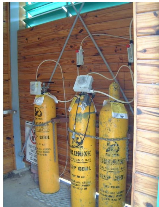
Chlorine Room Showing Cylinders and Chlorinators
