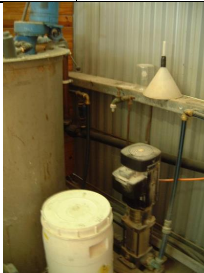
Photo of Polyacrylamide Batching and Dosing System
