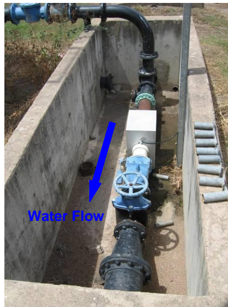
Photo of Pit on Treated Water Rising Main
