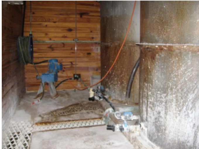
Photo of Alum Tanks and Pump (both unbunded)
