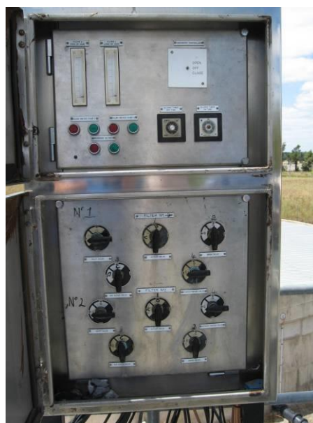
Photo of Filter Control Panel
