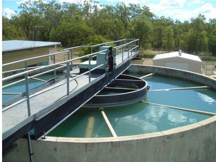
Photo of Clarifier Showing Central Flocculation Well and Settling Zone
