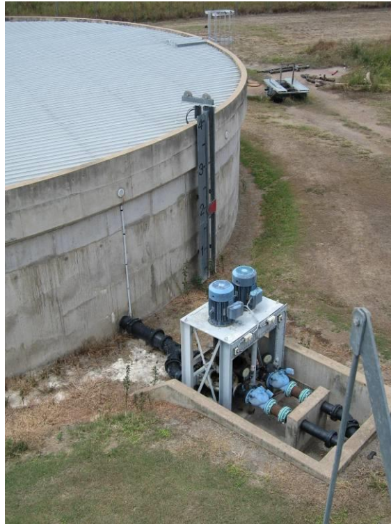
Photo of Clear Water Tank and Clear Water Pumps
