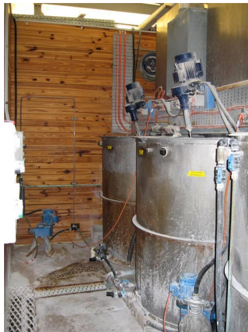
Photo of Alum Batching Tanks and Dosing Pump
