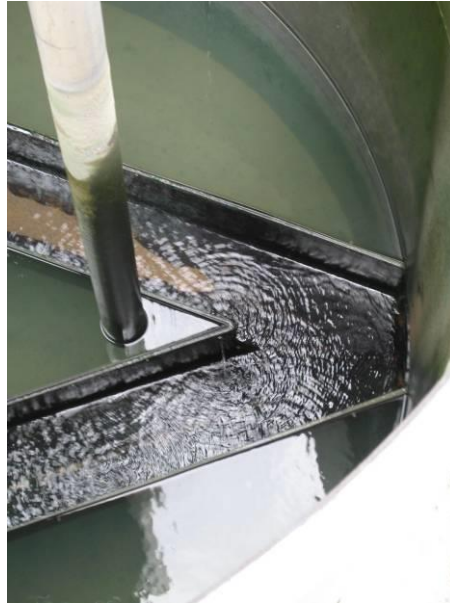
Photo of Filter 1 Showing Trough, PAC Dosing Tube and Media Surface
