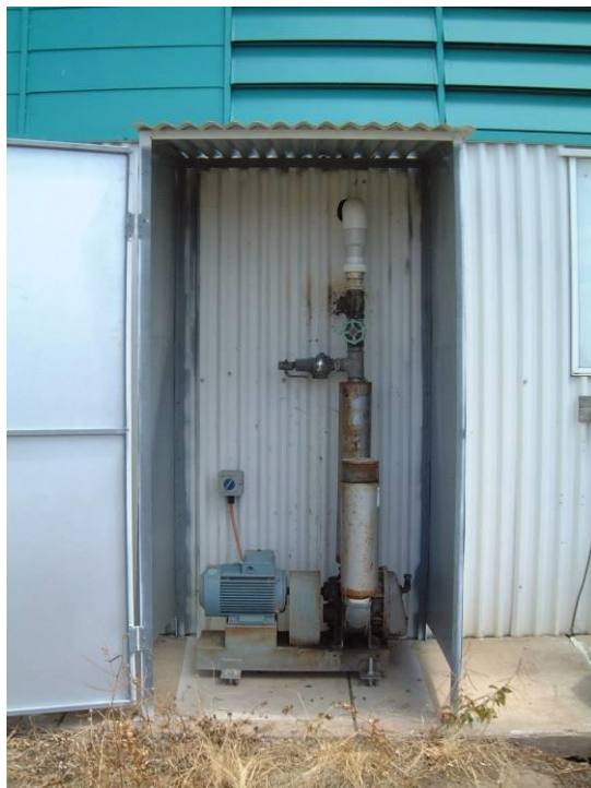
Photo of Air Scour Blower
