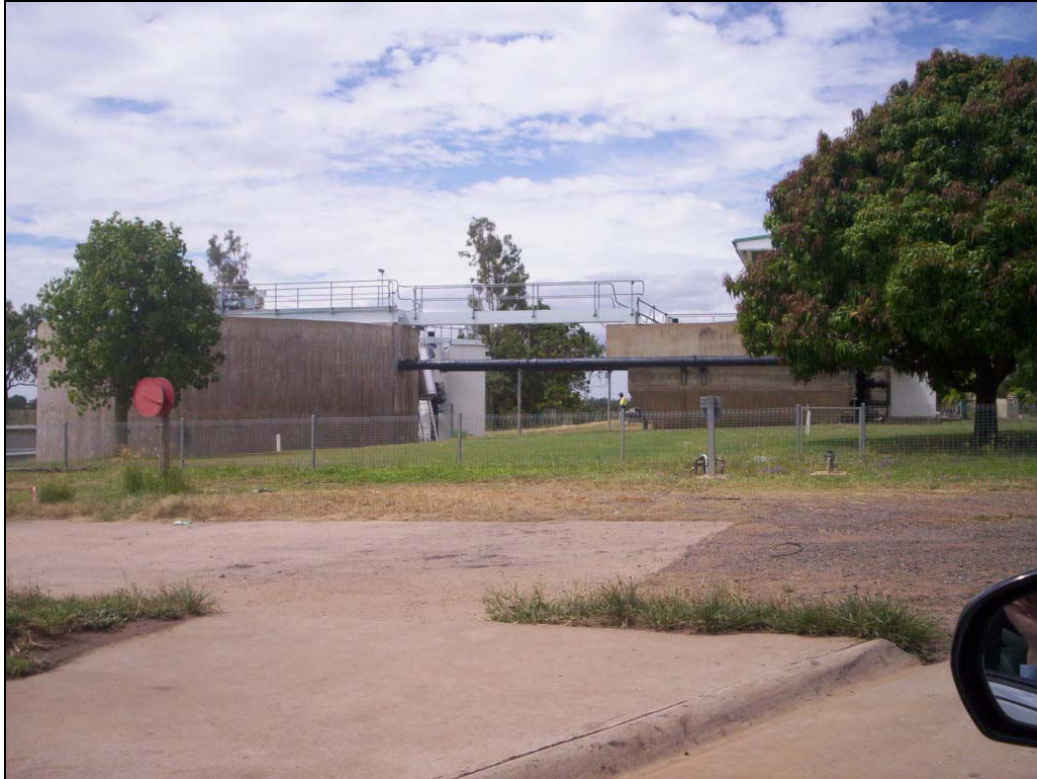
Figure A3 – Overview of Moura water treatment plant clear water storage tanks
