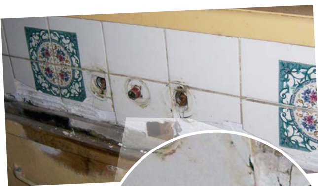
Ceramic tiles on asbestos sheeting
