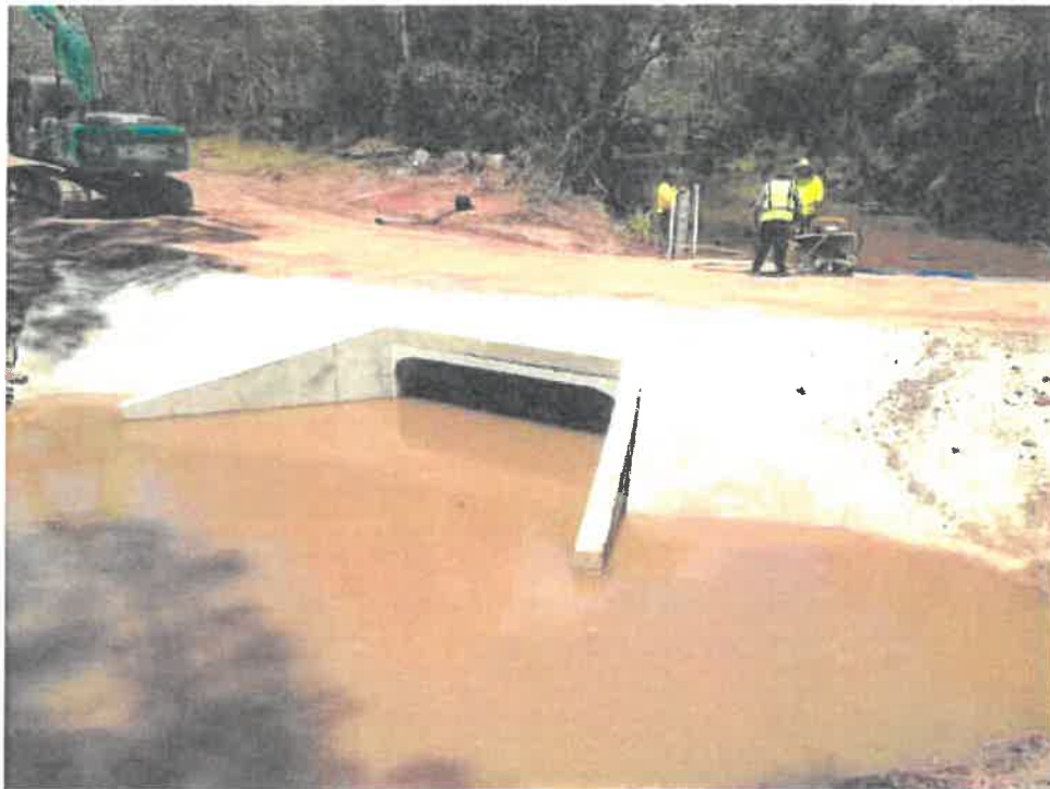
Photo D Looking at the completed waterway barrier works from a downstream position
