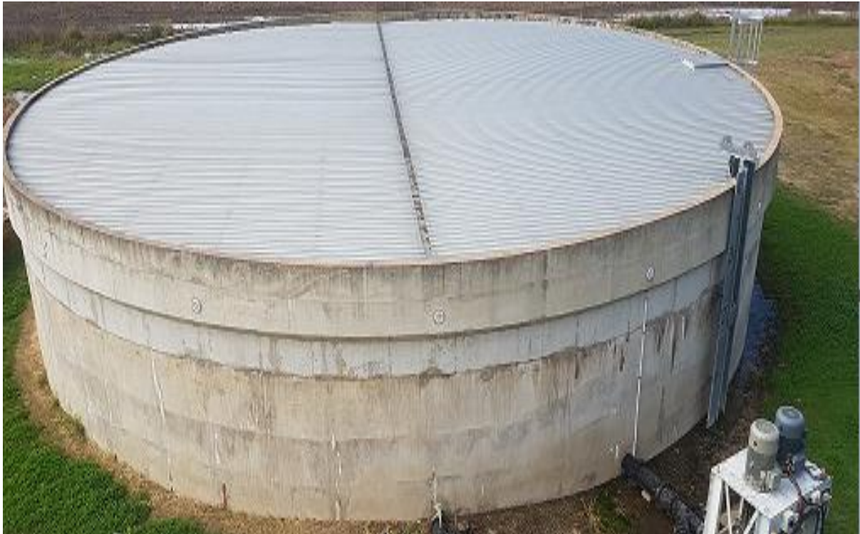
Figure 4: Aerial image of the Theodore clear water storage tank, of capacity 1.1ML; 21m dia., 4m high
