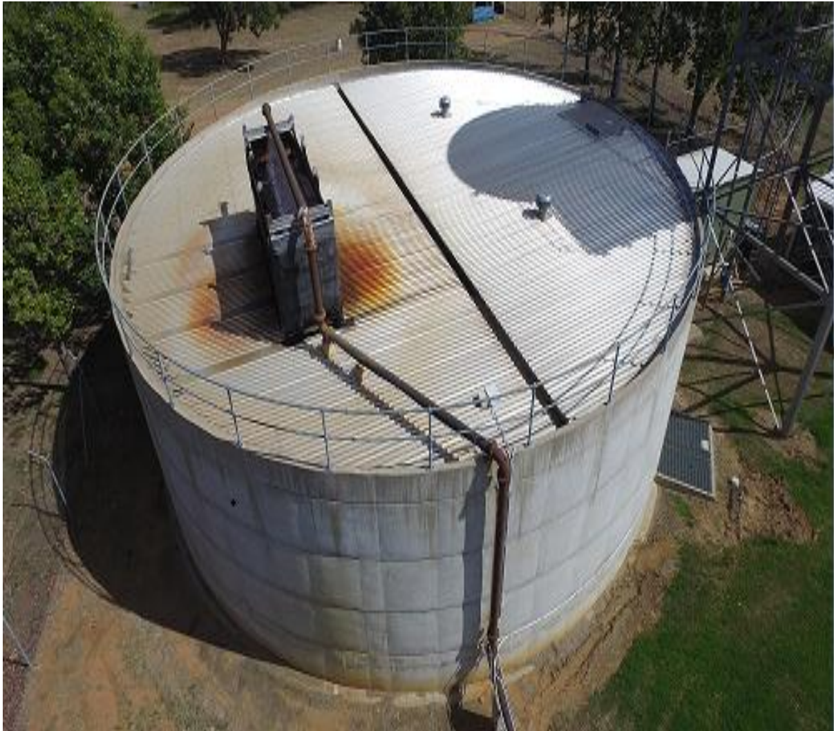
Figure 1: Aerial image of the Taroom water storage tank, of capacity 1.1ML; 18.4m dia., 5.45m high
