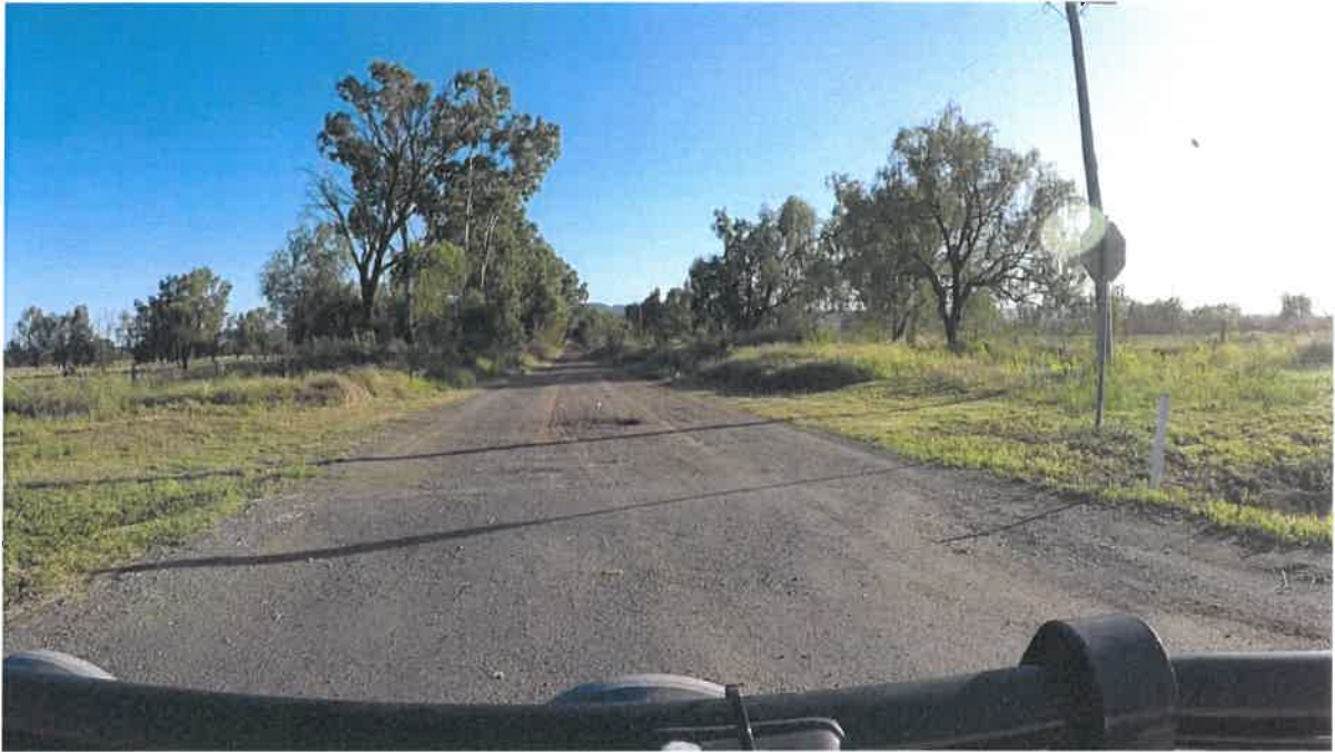
Figure 4-1 – Shorts Road Ch-02 – Biloela, QLD (Fatigue cracking above culvert – Sealed intersection)
