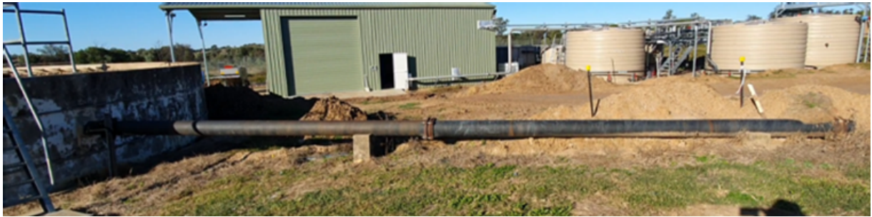
Figure 5-6 - Trickling Filter Inlet Pipe
