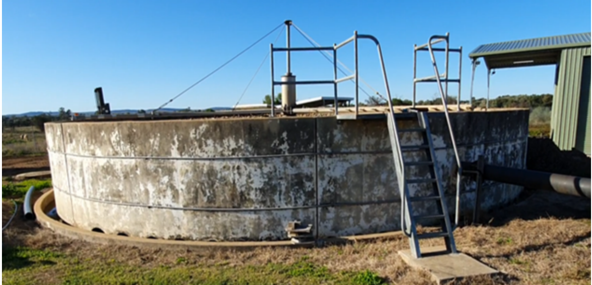
Figure 5-5 - Biological Trickling Filter Access Structure
