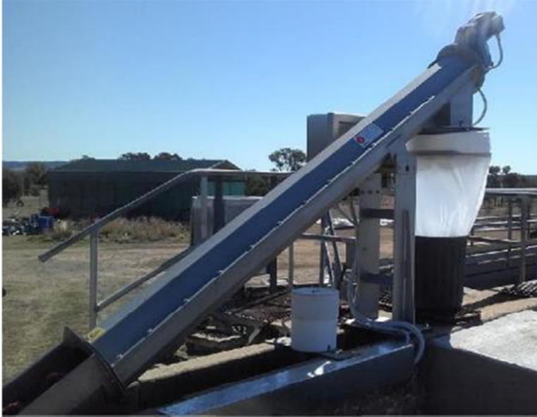
Figure 5-1 - Existing Inlet screen
