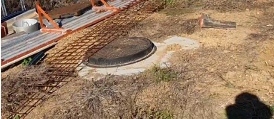
Figure 8 – 1050mm dia. scour pit within proposed swale.
