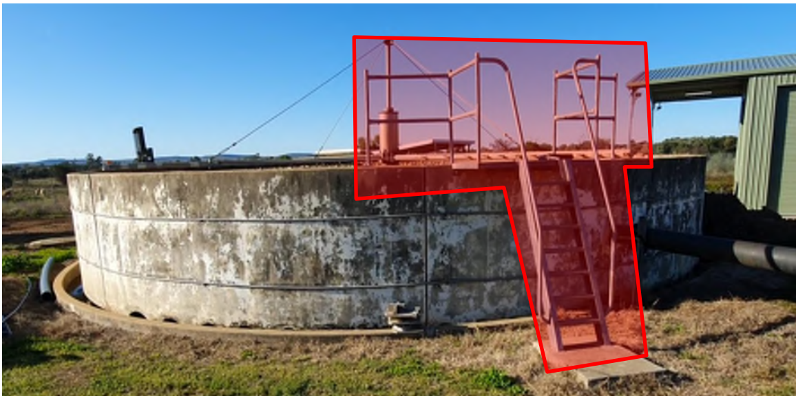
Figure 5 – Tricking Filter Access Structure
