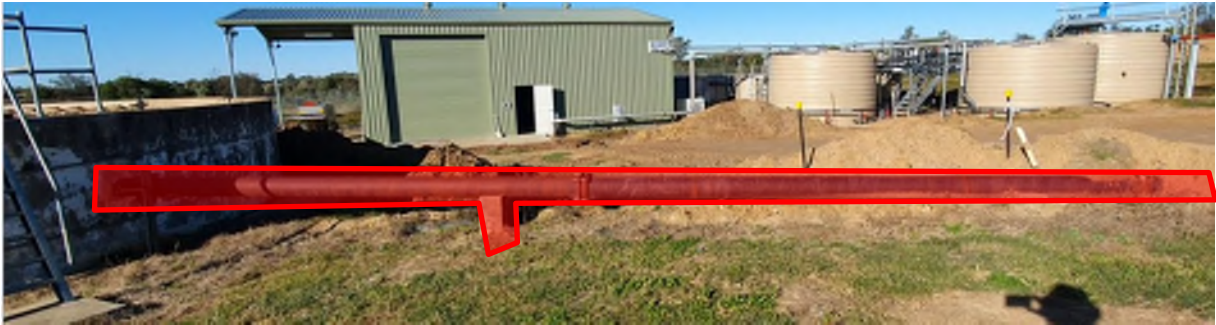
Figure 6 – Tricking Filter Inlet Pipe
