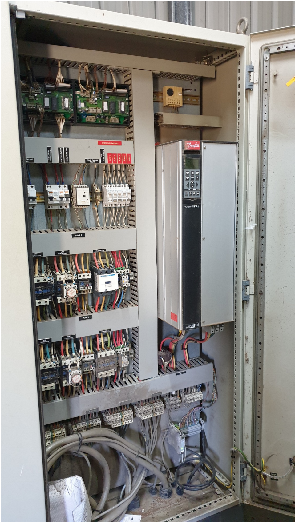
Fig 3- Existing Switch Board
