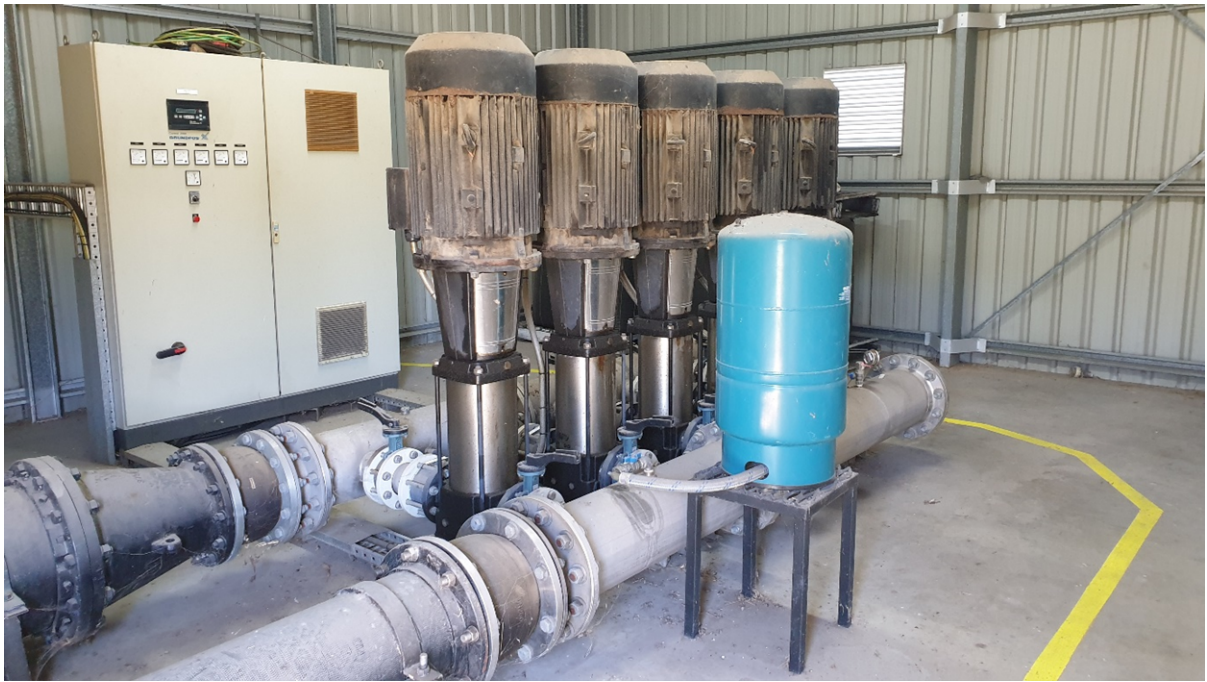
Fig 2 – Existing Booster set
