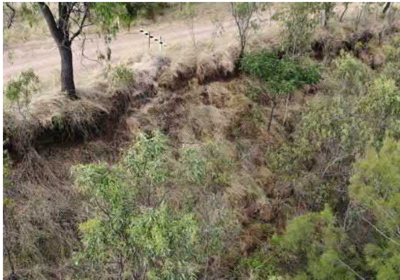
Figure 4 – Photo showing the geotechnical failure of the batter immediately adjacent to Kelly's Road
