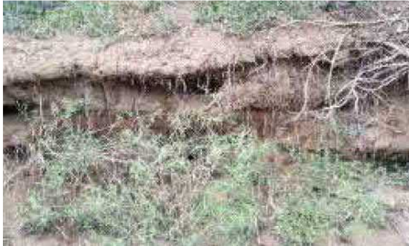
Figure 3 – Active erosion of the toe of the batter
