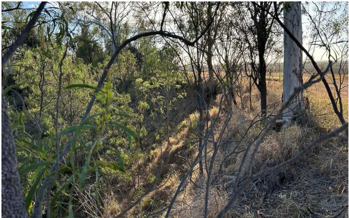
Figure 2: View of riverbank failure
